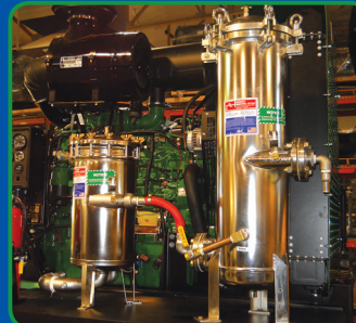
Organic material and particles filtered from fresh water to ensure high quality inlet water for the UHP pump.
